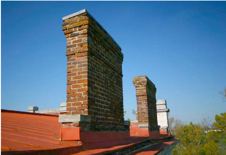
Figure 30. Two of the three East side chimney stacks. Photo, Anthony Eardley, October 2007
