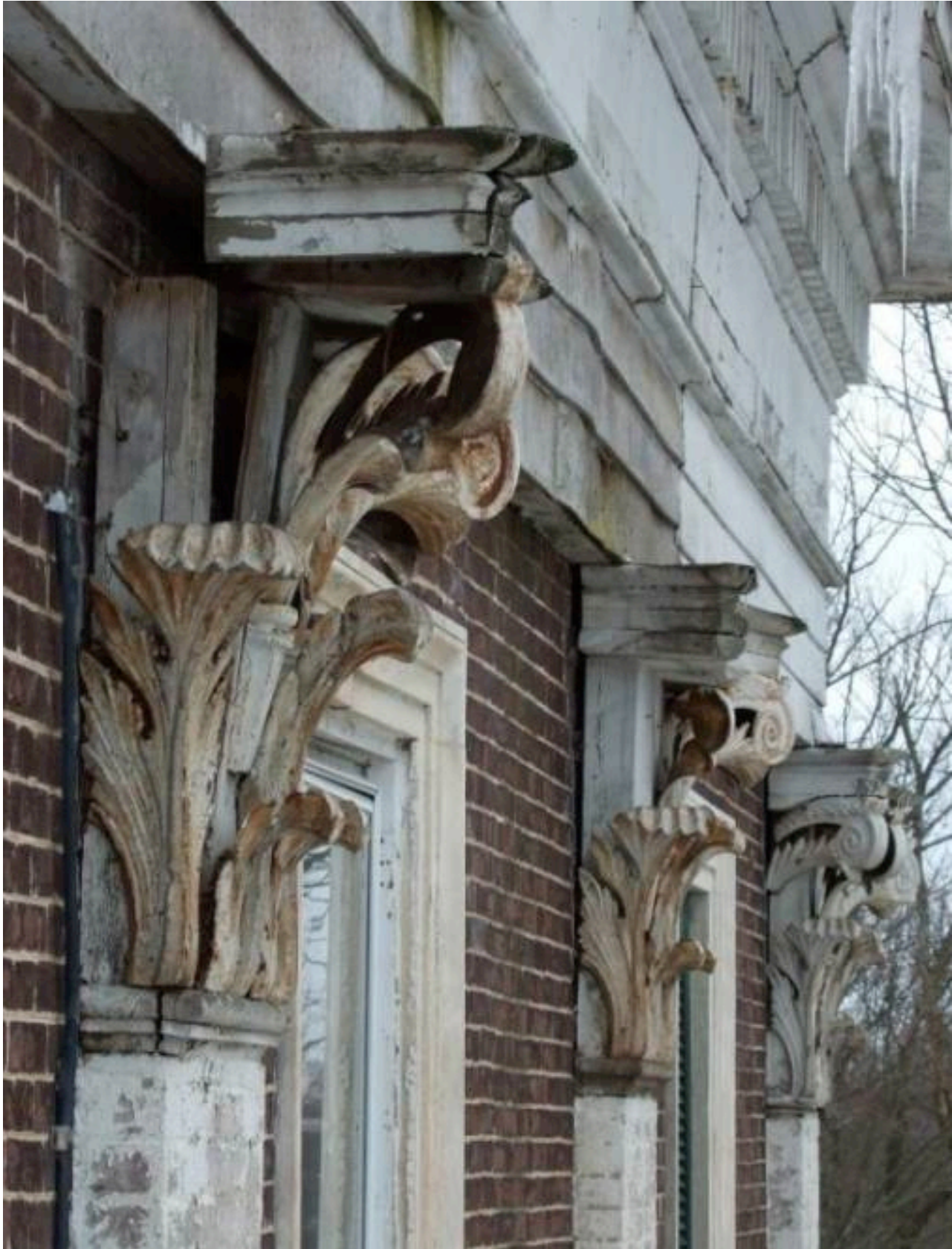
Figure 45. A 2007 view of the worst deterioration of the pilaster capitals on the West façade, the closest of which is now entirely disintegrated. Photo from Alison Brown, Conservation of the Cast Iron Pilaster Capitals at Ward Hall in Georgetown, Kentucky, Spring 2007
