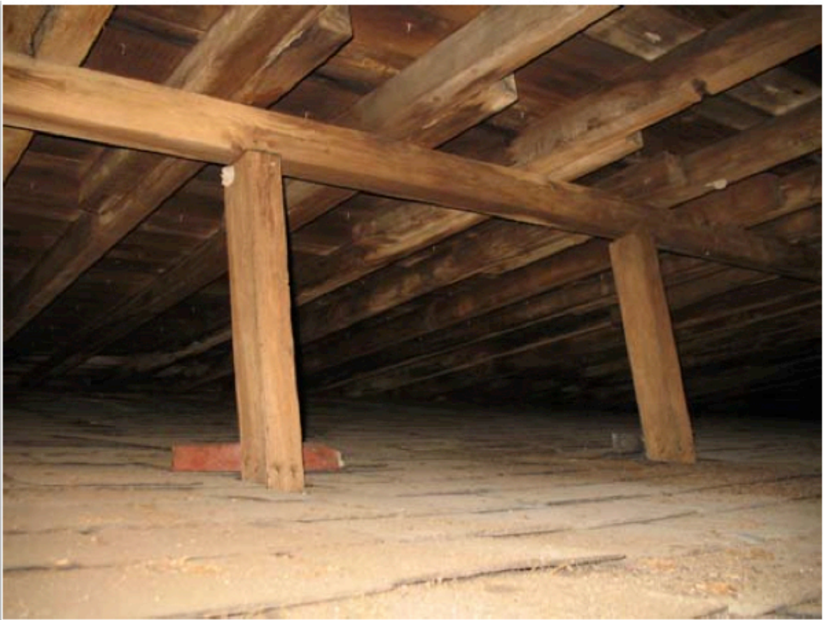
Figure 34. This shows the rafters of the second roof lying overlapped across a mid-slope purlin, which bears on posts supported by the original slate roof. Photo, Jerry Fryer, Structural Inspection Report, Revised December 5, 2008, BFMJ Structural Engineers, Lexington, Kentucky.
