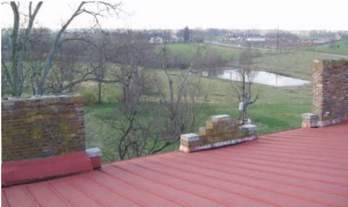
Figure 35. View across the Western slope of the second roof, showing the impediments to drainage created by the chimney stacks. Photo, Kentucky Heritage Council Report, December 2004, figure 78
