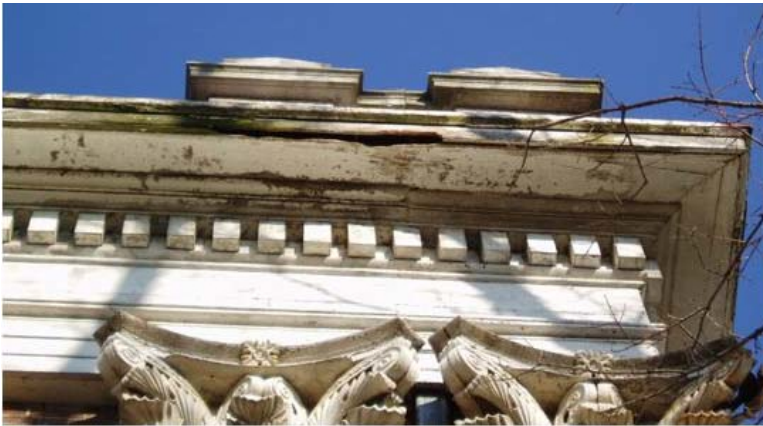
Figure 32. The underside of the cornice at the southeast corner. Photo, Kentucky heritage Council report, December 2004, figure 12
