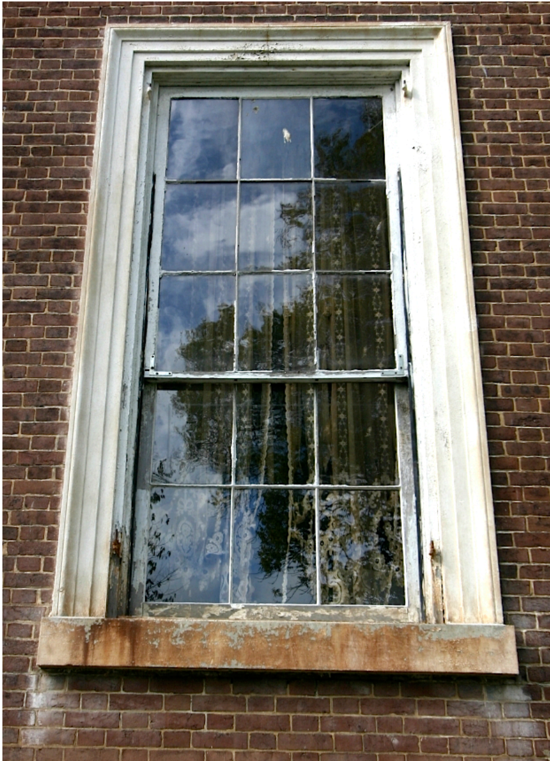
Figure 46. A nine over six double hung sash window in the East façade of the building, exhibiting typical problems of painted stone architraves staining the brickwork beneath the sill, paint loss to the woodwork, glazing putty loss, and failed frame connections to deteriorated bottom rails. There are no operable shutters to be found for these East and West side windows. Photo, Anthony Eardley, October 2007
