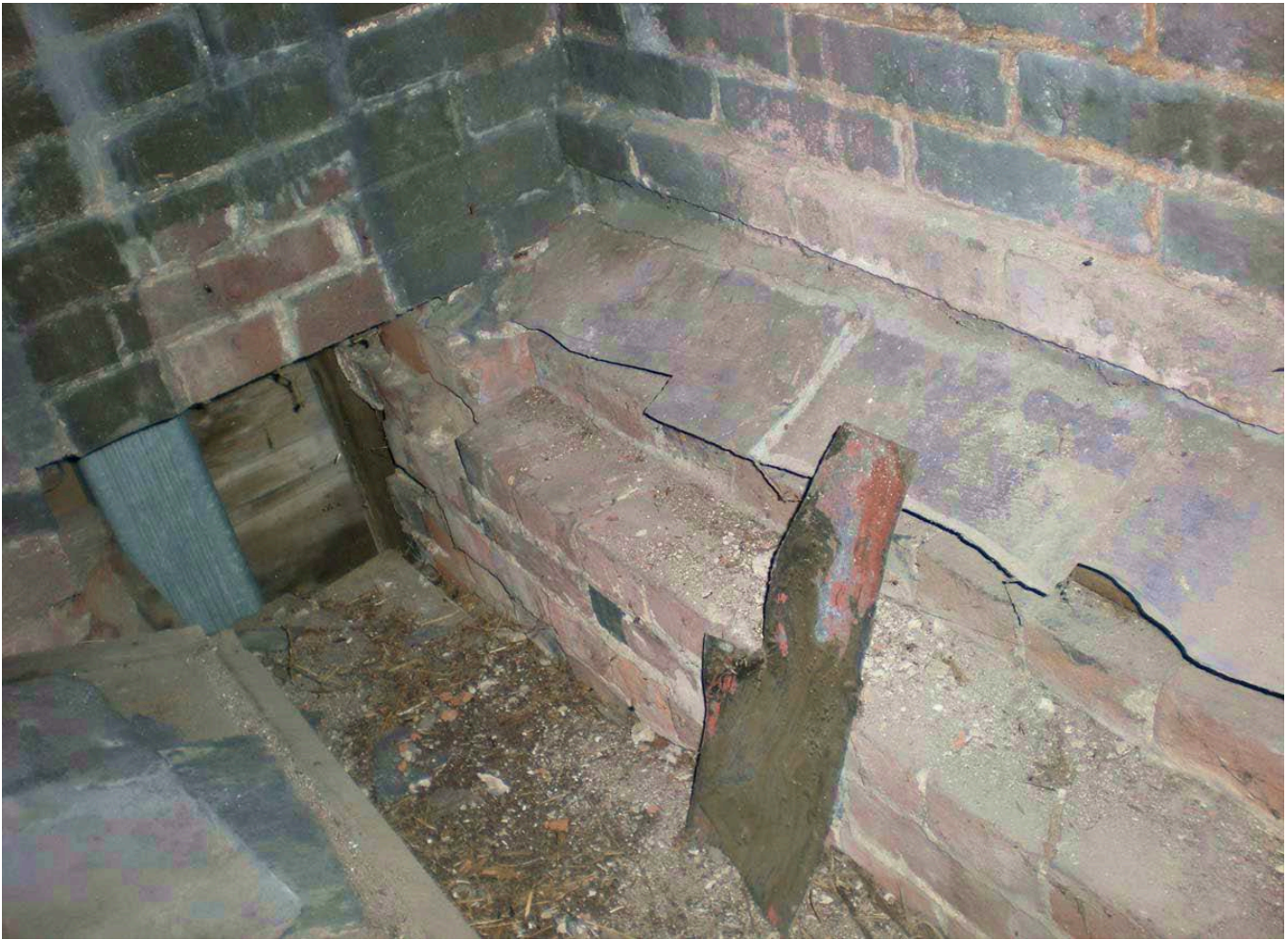
Figure 33. The hopper end of one of the original gutters running inside the East and West parapet walls, stripped of its lead lining some time after the installation of the second roof above it. Note the contrast between the soot-grimed walls, exposed to chronic downdraft smoke effects for perhaps the first twenty years of the life of the building, and the clean, formerly protected brickwork to the outside of the gutter. Photo, Geoffrey Bell, November 2008
