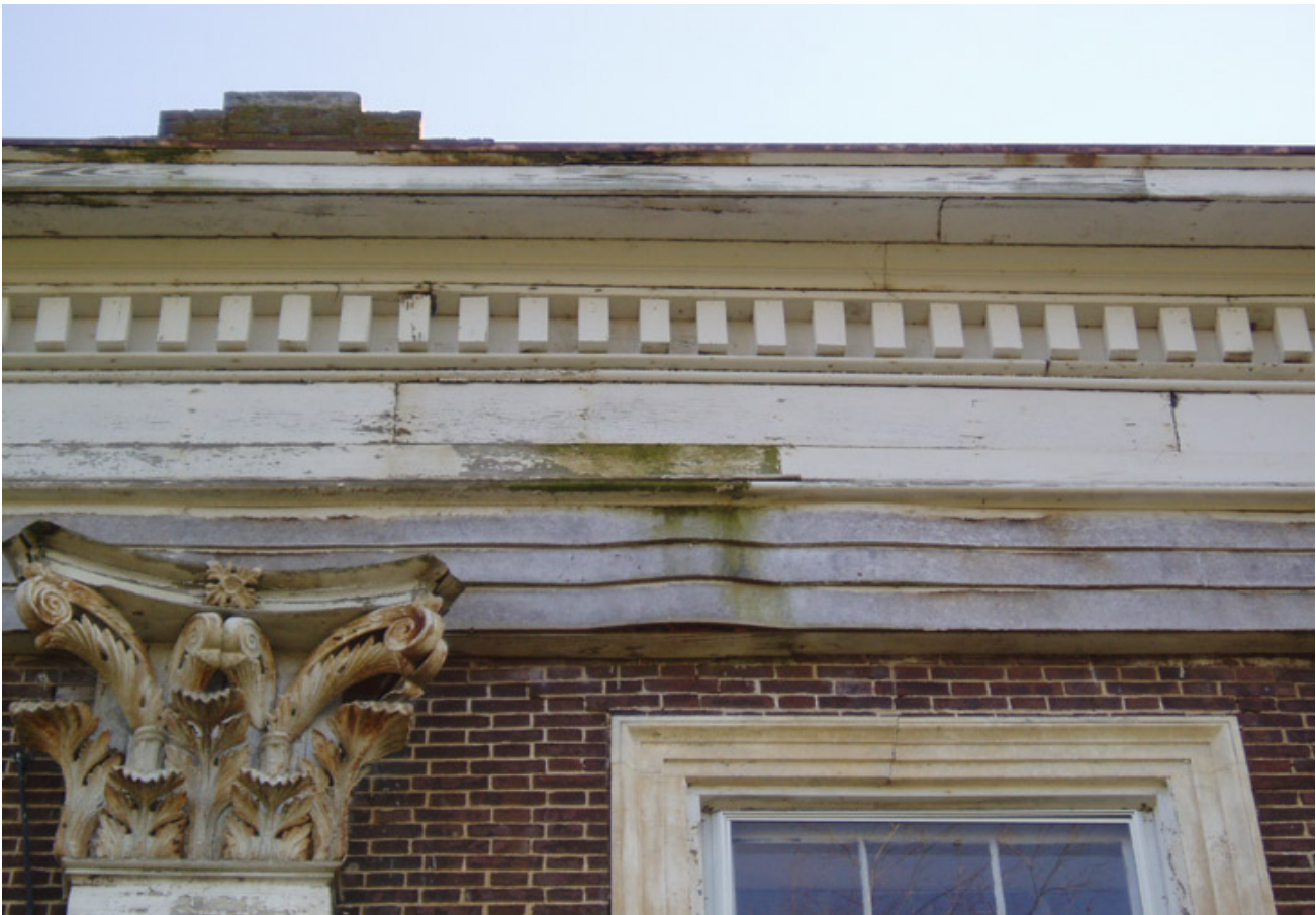
Figure 42. An example of past entablature repairs with inappropriate and inferior materials. Photo, Kentucky Heritage Council Report, December 2004, figure 7
