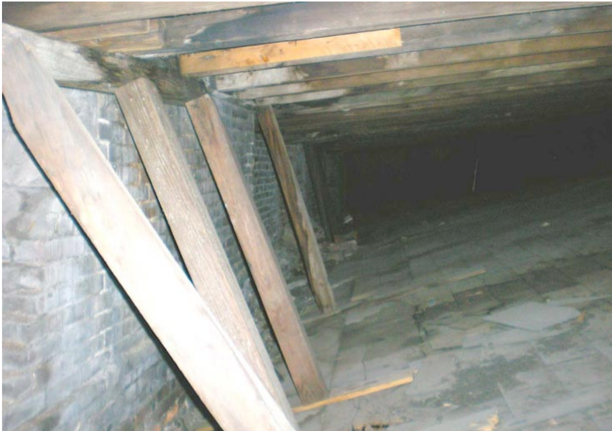
Figure 36. The space between the first and second roofs, showing the shoring typically necessitated by the failure of the upper roof structure at the chimney stacks. Photo, Geoffrey Bell, November 2008
